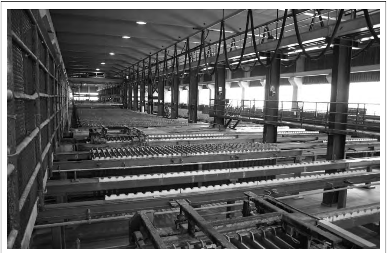
Figure 10: Cell house with two rows of 53 cells each
